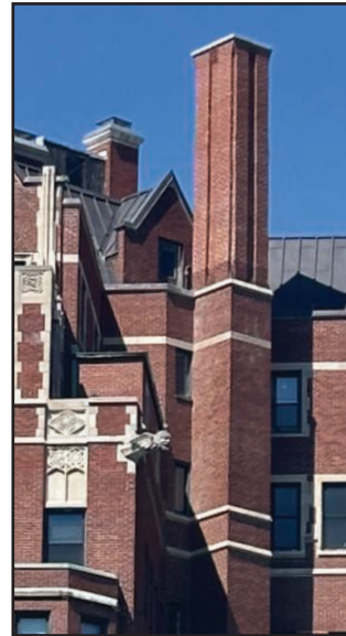
Before and After – International Chimney's Crew Rebuilding Chimney at Historic Downtown Buffalo Apartment Building
